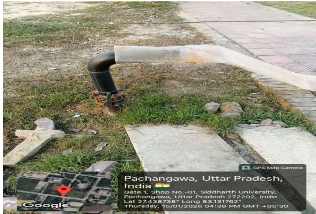
Watering the plant with recycled STP water
